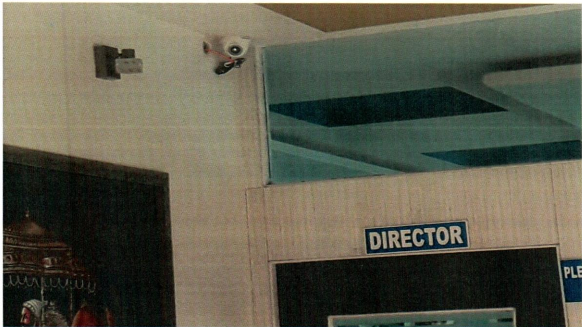
CCTV Cameras installed at various places in Institute
